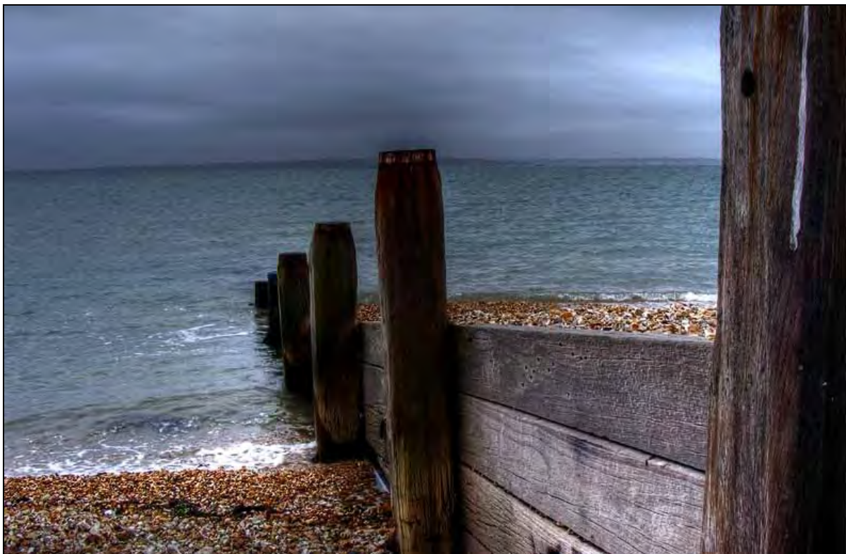
Figure 14: Example of Timber Groin, where Lagging can be Readily Removed or Added to Adjust Height
